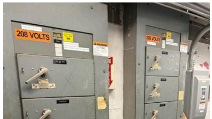
1960s electrical distribution panels
